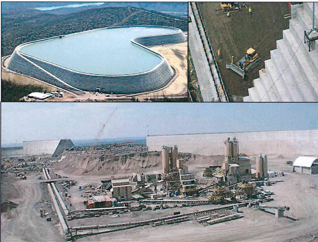
Picture 1: Taum Sauk Plant Upper Reservoir Dam (MO) RCC Placement and On-Site Aggregate Processing and Batch Plant
