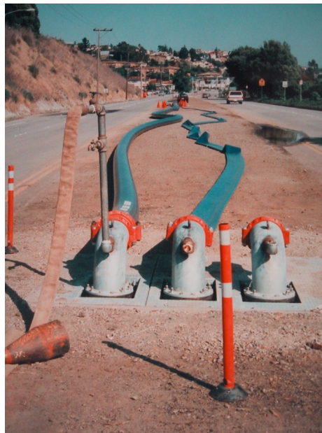
Figure 3. Flex Hose Attached to Manifold Outlets
