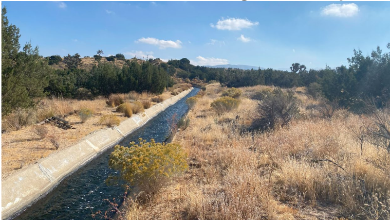
Photograph 1. View southeast of Palmdale Ditch approximately 425 feet east of 47 Street E undercrossing.
