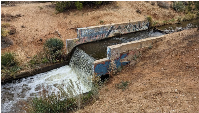
Photograph 3. View north of Palmdale Ditch approximately 2,700 feet east of State Route 14 undercrossing.
